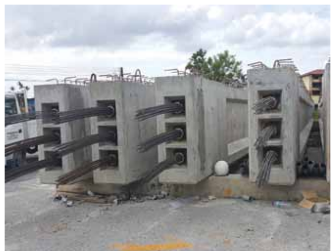
Post tensioning beams with anchor block and strand in place ready for stressing.
