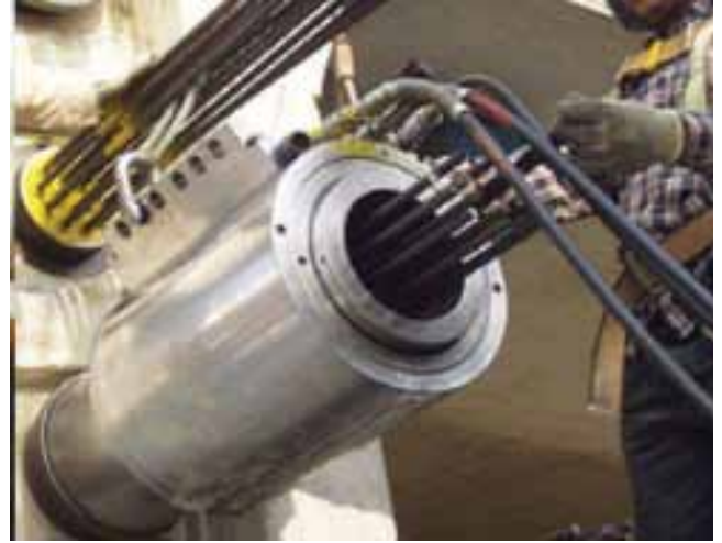
Multi Strand Stressing in progress. This process shall be done with caution.
